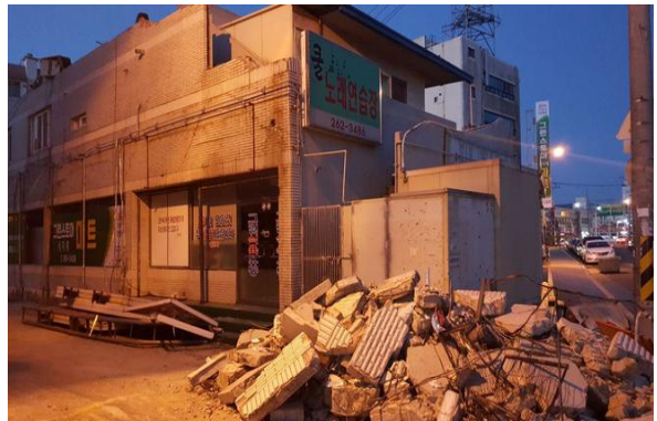
(b) Destruction of building wall
